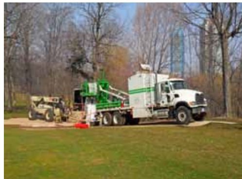
Capital Sewer Services used an EcoTek styrene-free resin for its ultra low VOC content.
