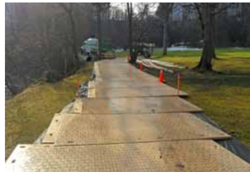
Access matting helped workers reach the job site and protected the terrain during repair.
